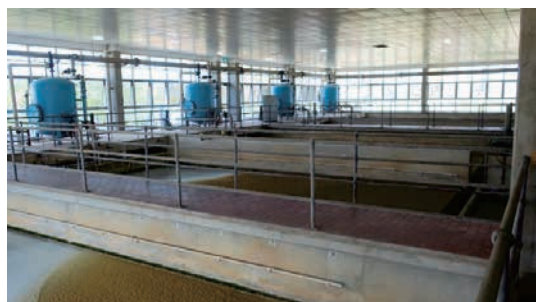
加圧浮上処理池 (DAF : Dissolved Air Flotation)
